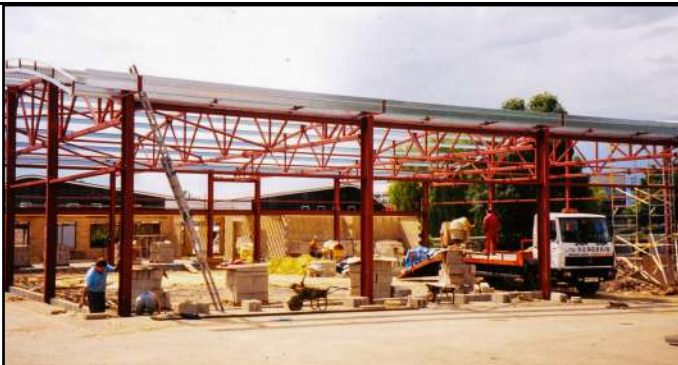
The steel frame and roof girders form the shape of the playing hall
